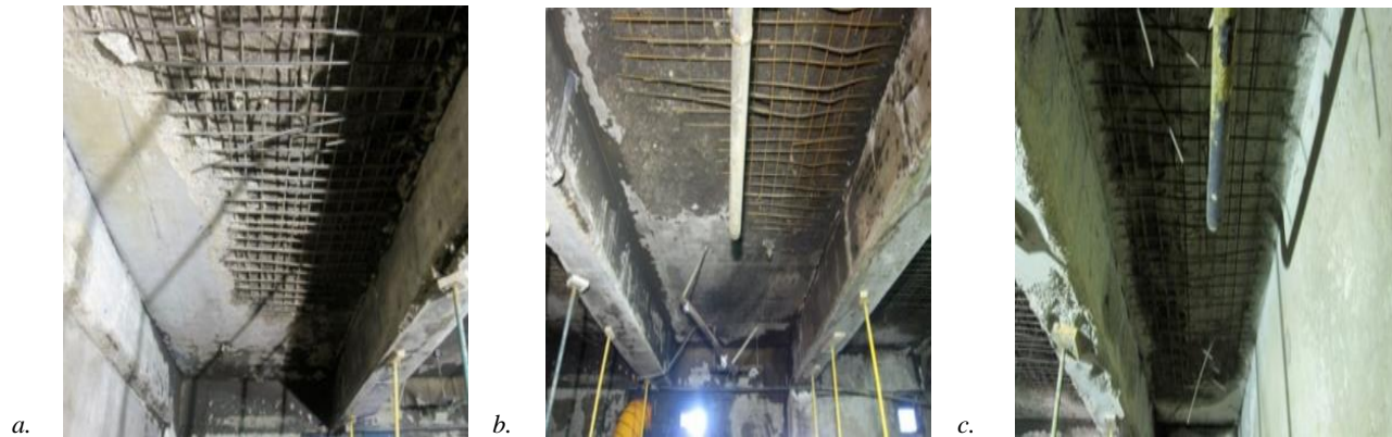
Figure 2. Destruction in slab soffit: a. Slab#1, b. Slab#2 and (c) Slab#3 [10].
