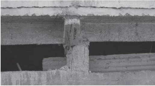
Figure 3: Shear failure in RC short column [1]
