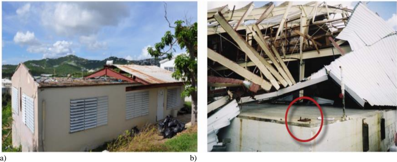
Figure 4: a. Wind induces damage to steel frame structure, a. collapse of steel roof frame during hurricane Irma and Maria, 2017 [32] and b. roof frame failure and gable end wall collapse due to insufficient latera support during hurricane Hurrucane Charley, 2004. [33]
