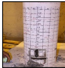
Figure 3. Damaged Column, Cracks & Spalling of concrete.
