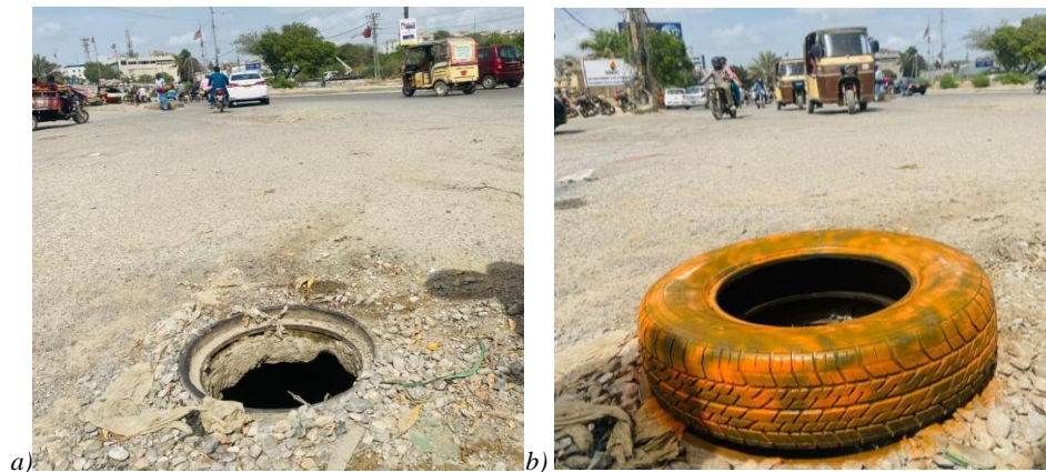
Figure 3: a) before the installation of rubber tire, b) after the installation of rubber tire.
