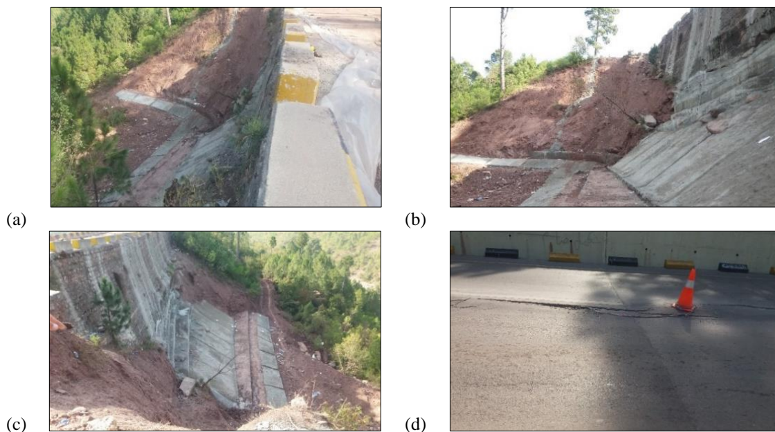
Fig. 2 (a), (b), (c), (d) shows top, right side, left side and road view (with tension crack) of slope
