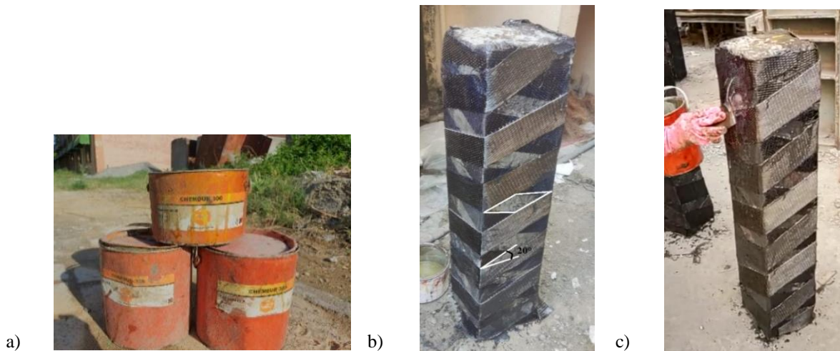
Figure 1: Preparation of specimen, a. CHEMDUR 300 (component A and B), b. Covered column by CFRP strips at 20°, and c. Applying bonding agent on column.
