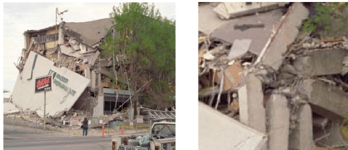
Figure 1: Building collapses due to beam-column joint failure [4]
