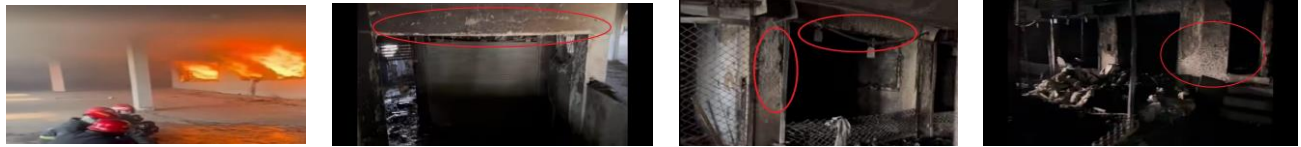
Fig.1: Damages to RC structure: a) RC structure under fire, b) Cracking, c) Cracking and loss of cover, d) Exposure of aggregate
