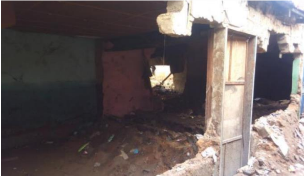
Figure 5 a: Partial Collapsed of Building [12]
