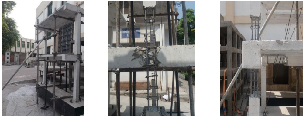
Figure 2-1: (a) Damaged Frame, (b) Damaged concrete removed from joints, (c) Joint after concrete removal
