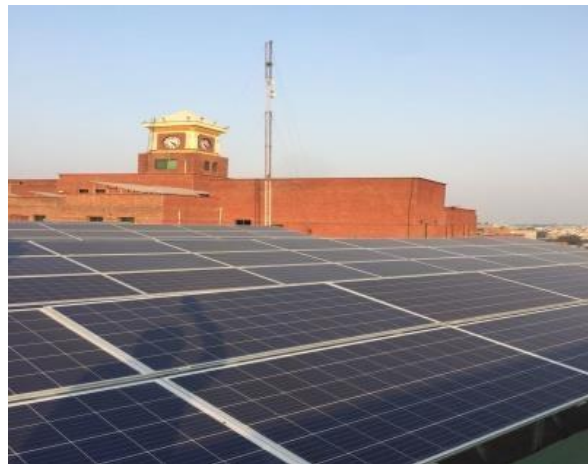
Figure 5: Solar panels installed on roof.
