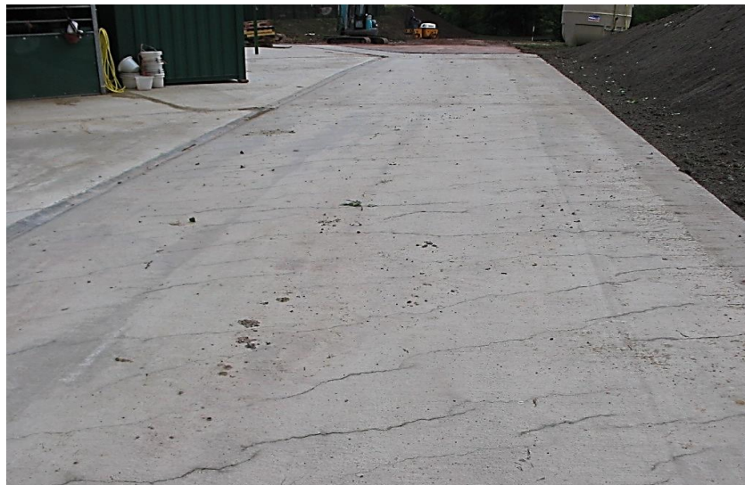
Figure 2: Shrinkage cracking in rigid pavement
